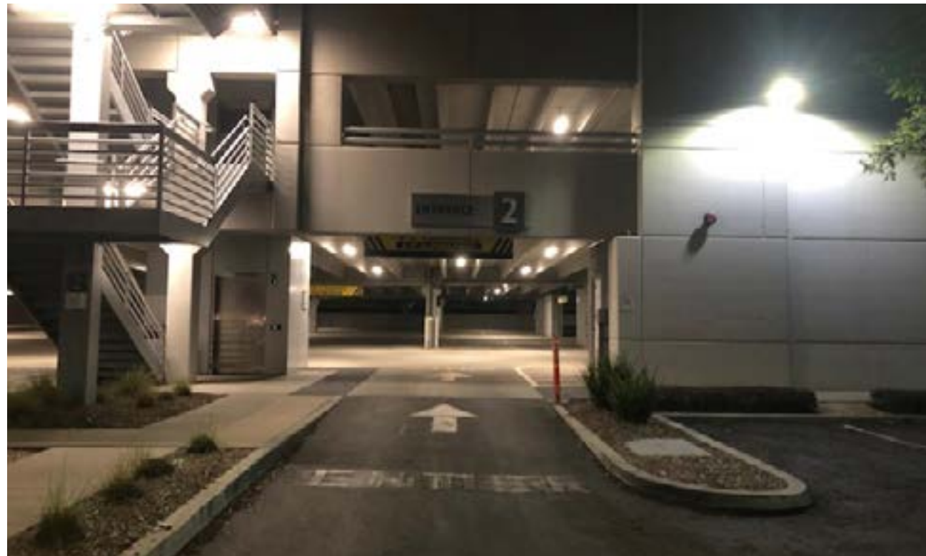
LED LIGHTING RETROFIT COMPLETED IN 2018 AT OUR PARKING GARAGE AT KILROY CENTRE DEL MAR, SAN DIEGO, CA
